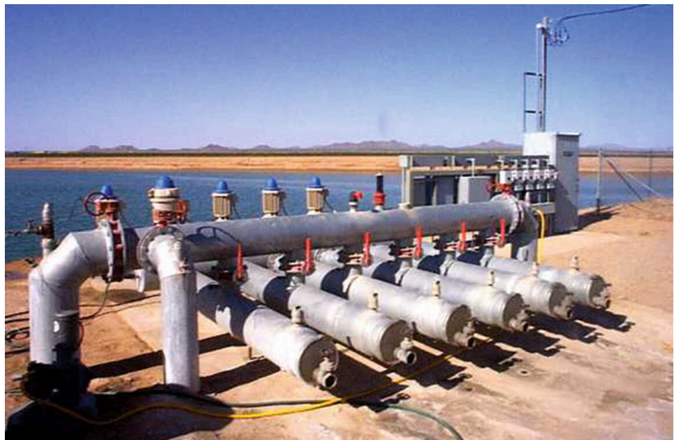
Fig. 12.30 Reservoir and pump station for center pivot farm. Cylindrical stainless steel ring filters and manifold in foreground. Motors on top of turbine pumps are seen behind manifold (Credit Paul Colaizzi, University of Arizona and USDA-ARS Bushland, Texas)
