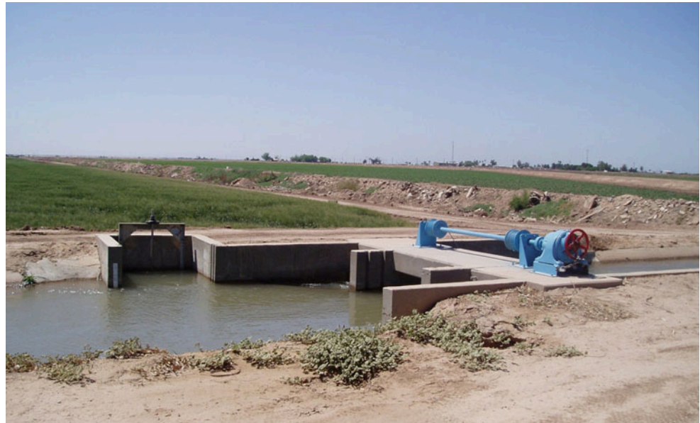
Fig. 11.3 Headgate on irrigation district lateral canal and downstream control structure
