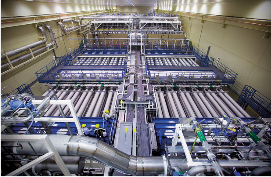
Fig. 10.60 The laser bay of the National Ignition Facility [courtesy of Lawrence Livermore Laboratory via Google Images]
