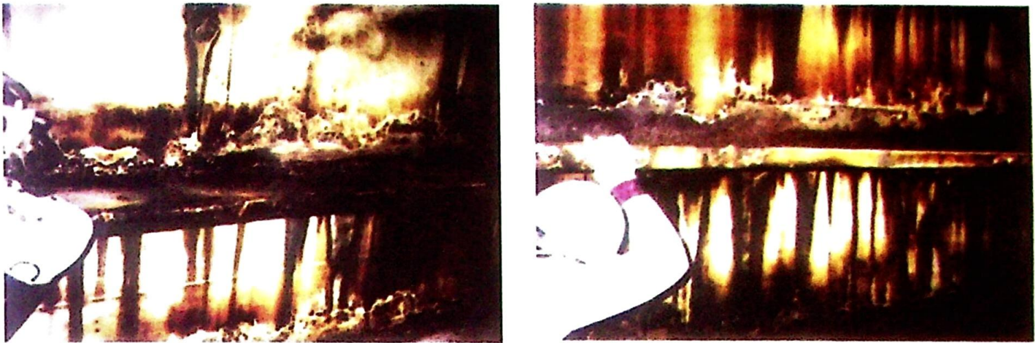
Figure 1.9: Corrosion of Longitudinal Bulkhead, Coated Segregated Ballast Tank
