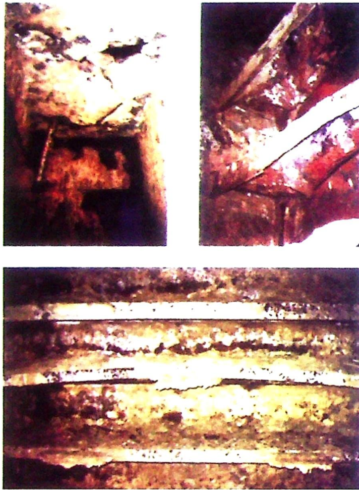
Figure 1.7: Corrosion of Longitudinal Bulkhead Longitudinal Stiffeners, Uncoated Segregated Ballast Tank
