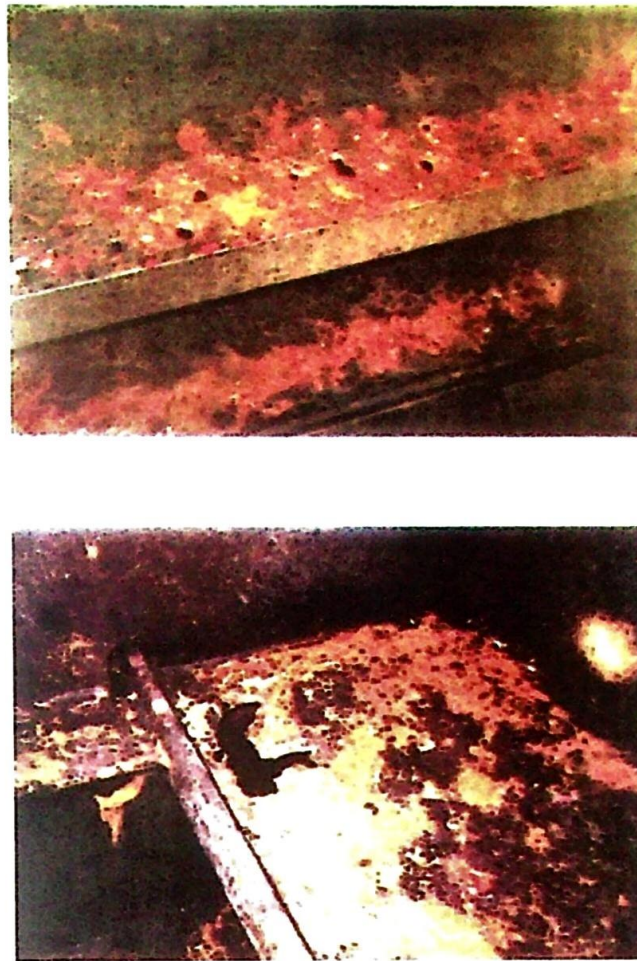
Figure 1.13: Corrosion of Side Shell Longitudinal (Uncoated Cargo/Departure Ballast Tank)
