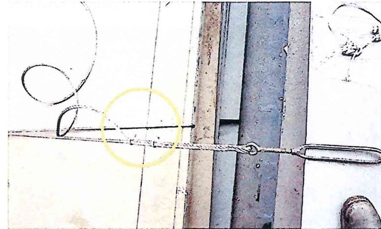
✗ The wire clips are insufficient and are also incorrectly placed. The saddle should be on the live wire and there should be a minimum of three grips
