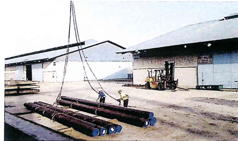
✓ 12" diameter pipes, bundled in pairs, pre-slung for tip-lifting and using nylon slings for a basket lift of eight pipes (four pairs)
