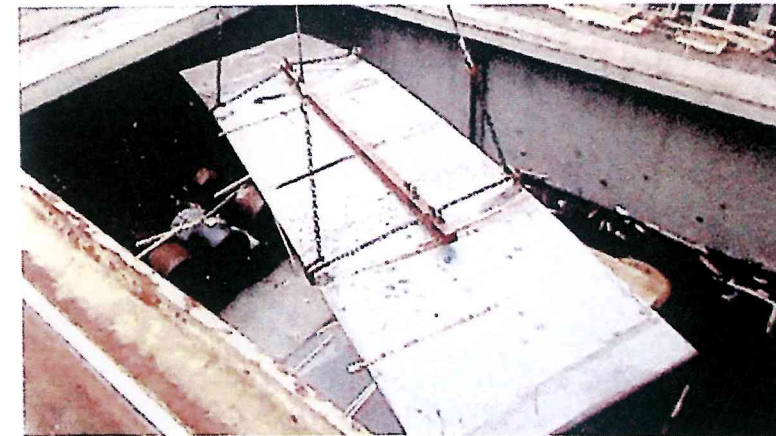
✓ Discharging of unbundled, unpacked steel plates. Use of 'C' hooks and a spreader
