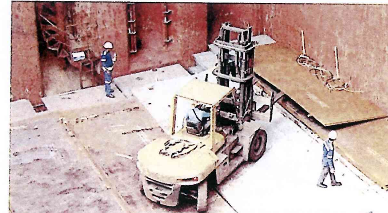
✗ The absence of dunnage between the plates creates extra work and also risks cargo damage in this process
