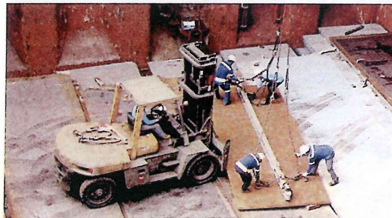
✓ The steel plate is pulled out of the under-coaming space for direct access with the crane
