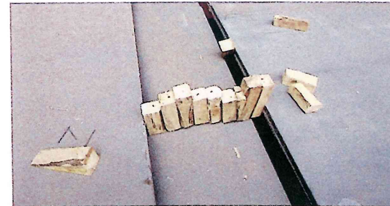
✘ Incorrect use of dunnage. The pieces of wood are prone to collapse. Whole pieces of dunnage should have been used in several locations for chocking
