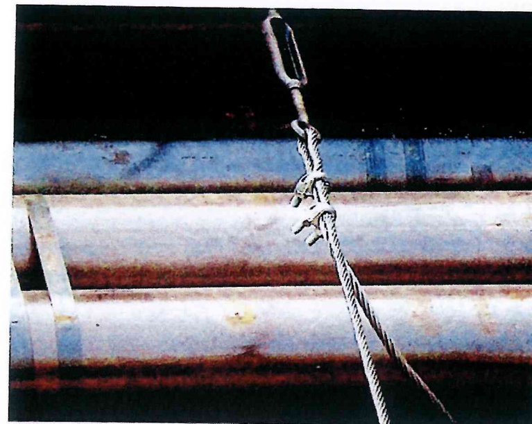
✘ Insufficient number of grips used and the saddle should be on the live wire
