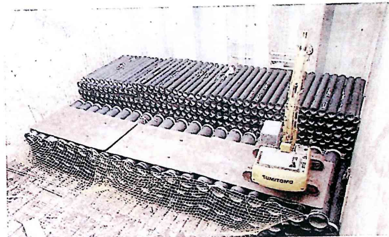
✓ Stows being built up in a safe and efficient manner. Steel plates have been laid across the pipes to protect them and to spread the load of the backhoe
